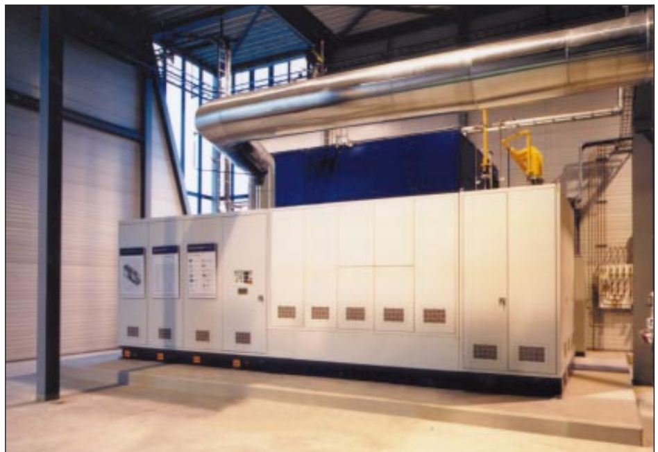
100-kW SOFC cogeneration system operating in The Netherlands, built by Siemens Westinghouse (photo courtesy of Siemens Westinghouse)
